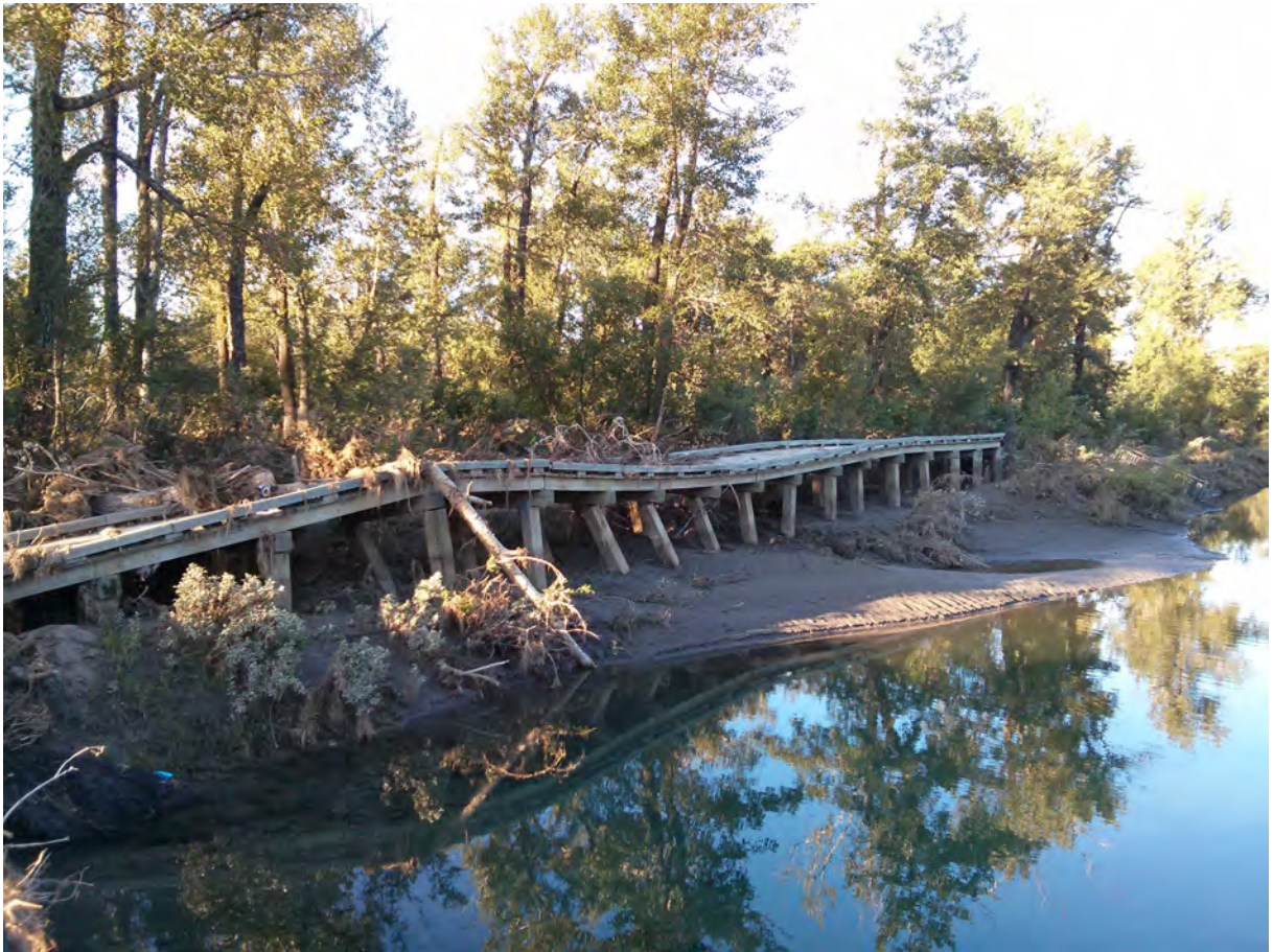
Aftermath of June 2013 Catastrophic Flooding
